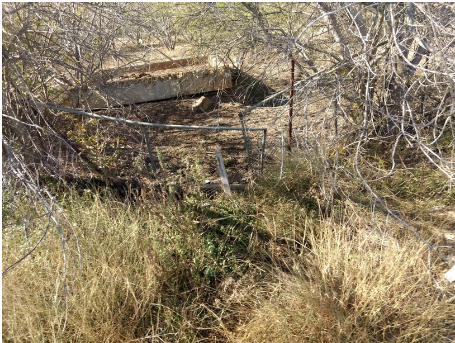
Photo 4: View into the subject site showing a large, apparently discarded concrete piece and dilapidated chain link fencing.
