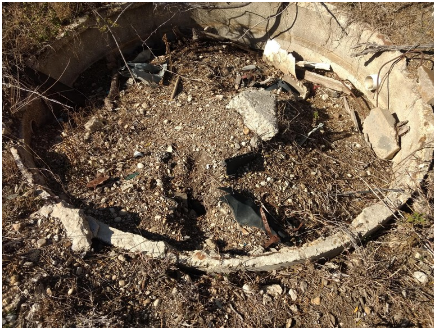
Photo 24: View of an apparent septic tank collapsed and filled in with dirt and debris observed near the vacant slab on the northeast portion of the site.
