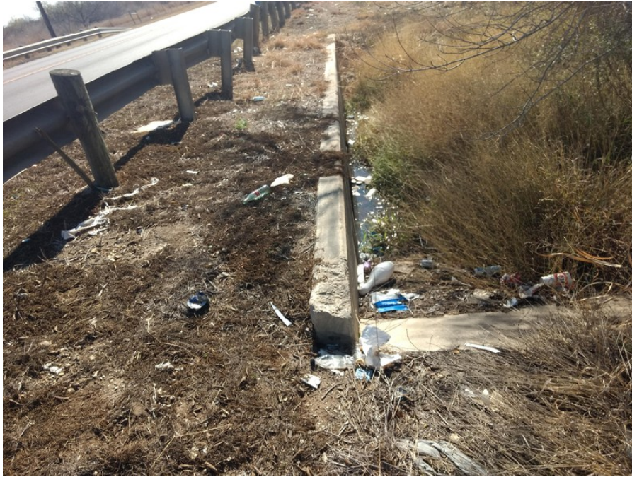
Photo 5: View into stormwater drainage channel showing trash and standing water, along Pleasanton Road.
